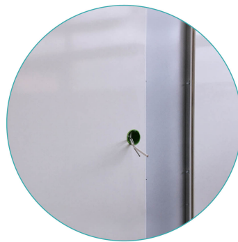
Uncovered installation panel and elektroinstallation
